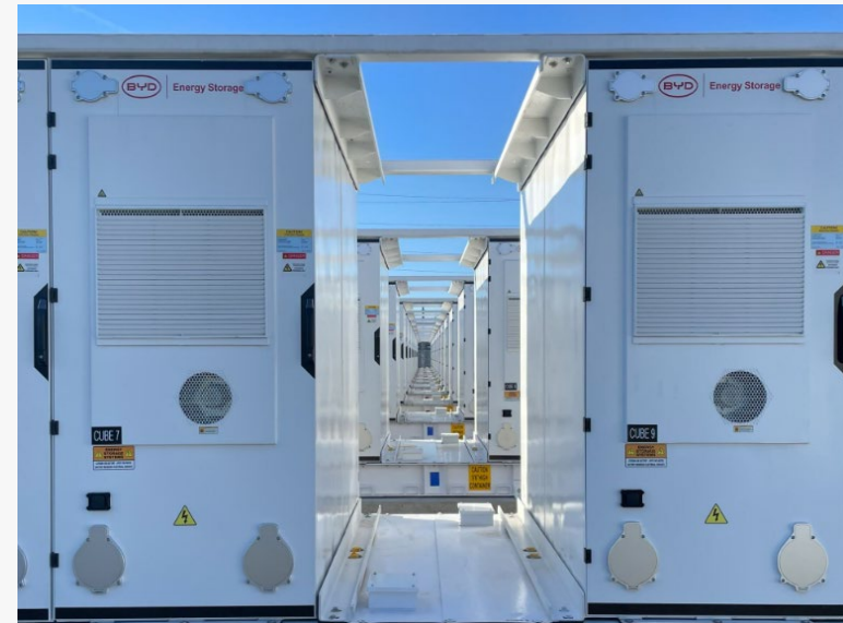
Constable Battery Energy Storage System
